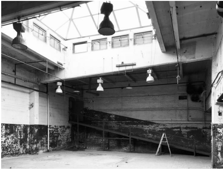
Phase Two Boiler Room
