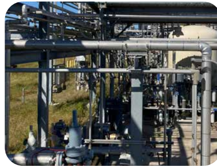
Several test structures on site were used to conduct tests related to pipe fittings.
