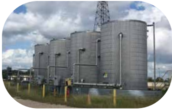
Rainwater Collection Existing Tanks
